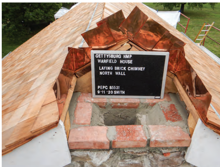
Detail of the restoration of the James Warfield home. NATIONAL PARK SERVICE
